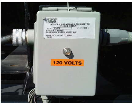
Over night heating system
